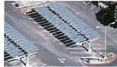
Solar parking lot canopies, such as this one at Cal State Northridge, are highly visible signals to consumers about the benefits of solar
