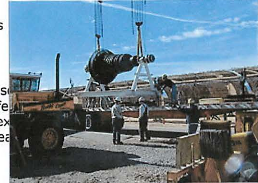
For standard overhaul, workers remove a 30-MWe steam turbine from the SEGS V power plant in Kramer Junction, California.
