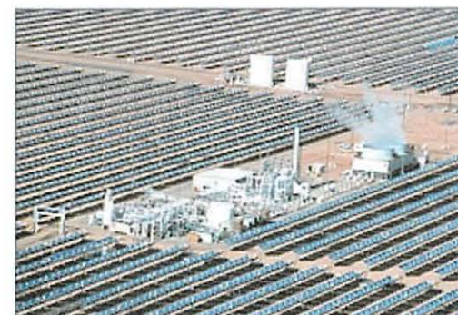
The SEGS IV parabolic trough power plant in Kramer Junction, California. Credit: Sandia National Laboratories
