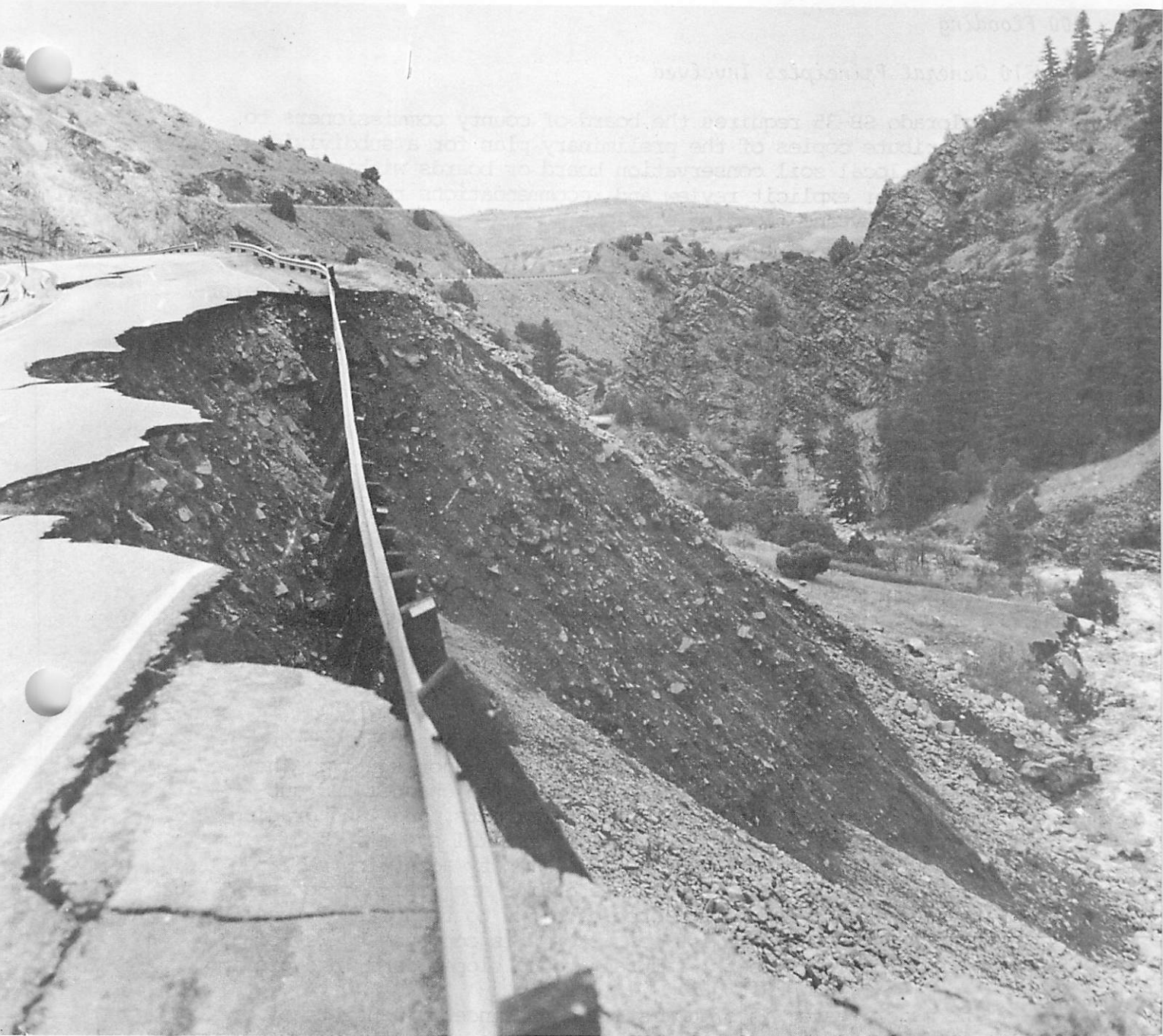
Drainage and soil suitability are important in road construction. SCS PHOTO 10-PI479-1
