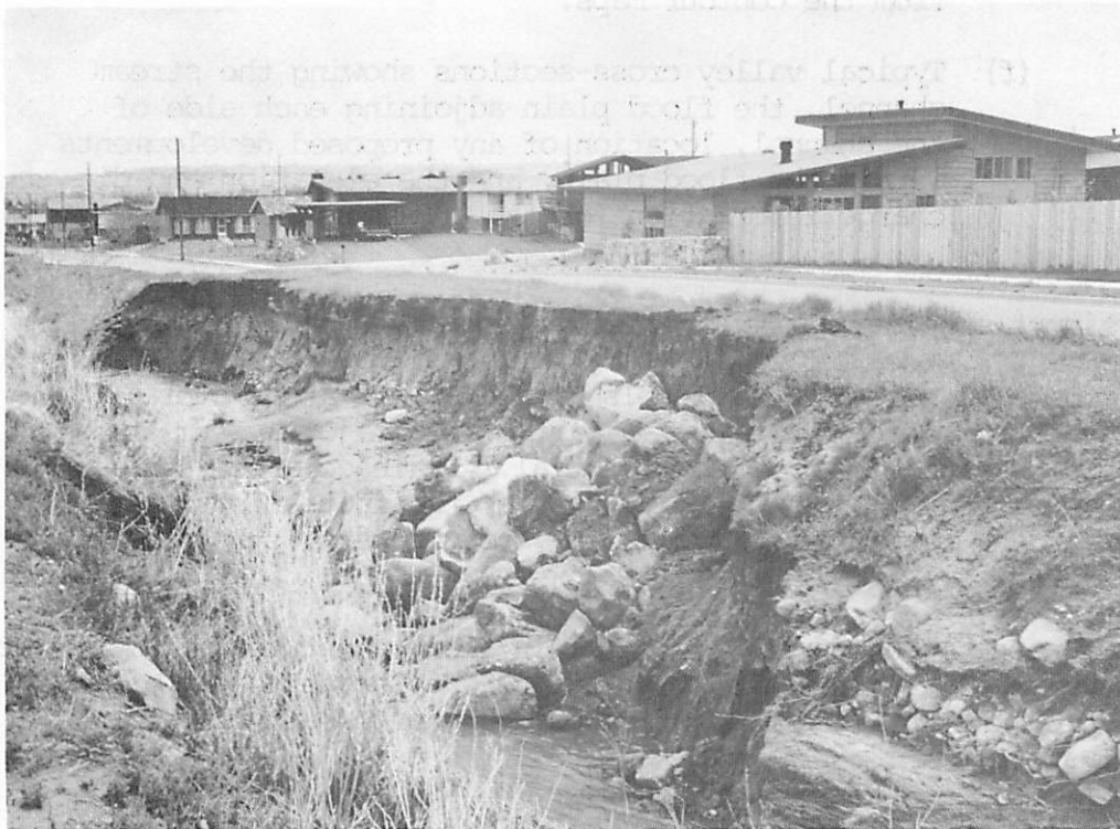
Runoff from developed area is too much for existing channel.
