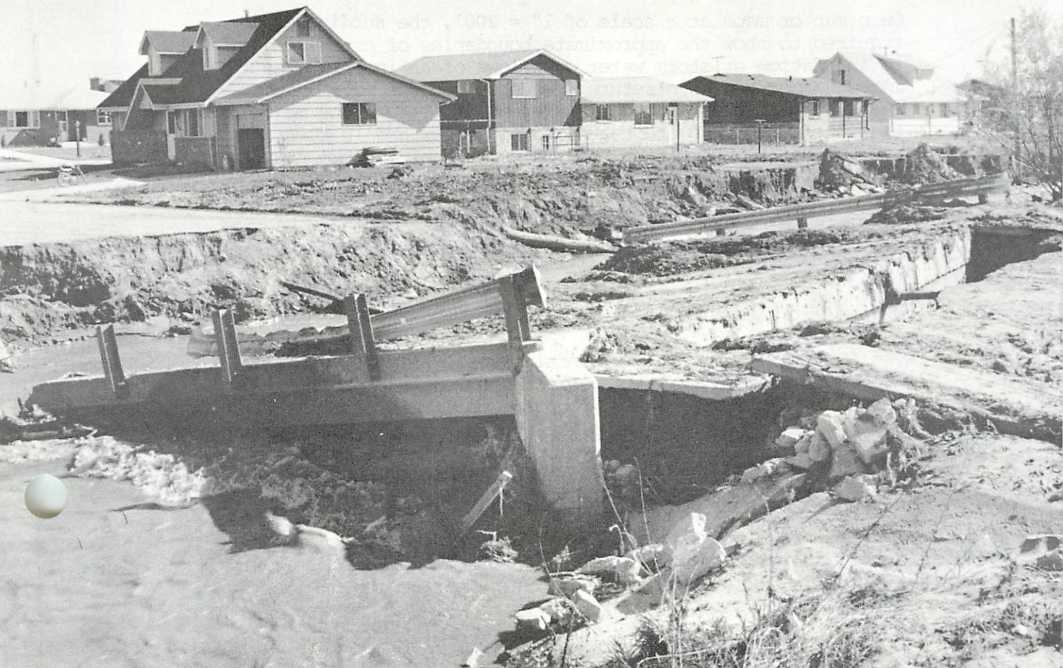
This bridge couldn't handle increased flow from development area. SCS PHOTO 10-P810-3
